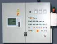
Electrical control panel
