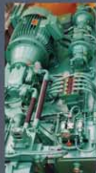
Hydraulic power unit
